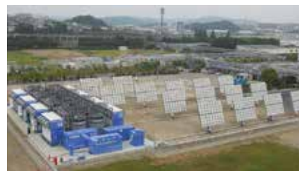
Figure 17: Flow battery storage system. The figure 17 show that the example for the Flow battery storage system which is the construct in the Japan for the store excess solar energy.
